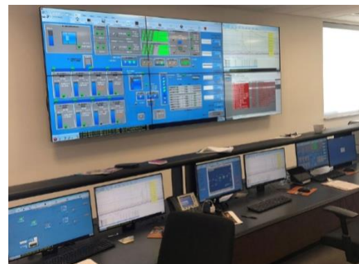
Figure 3. Monitoring room sample
