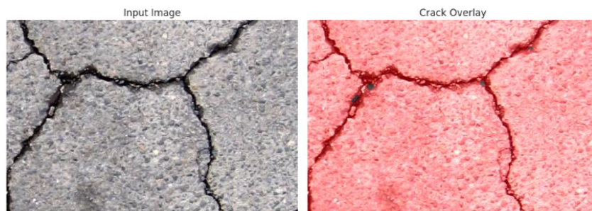
Figure 4. Road damage image overlay
