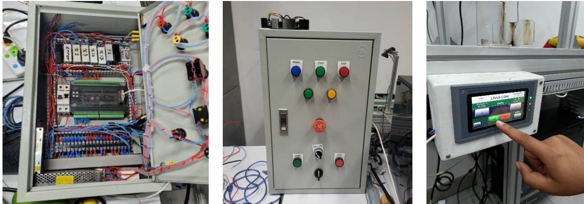
Figure 3. Automatic machine control panel with PLC and HMI
